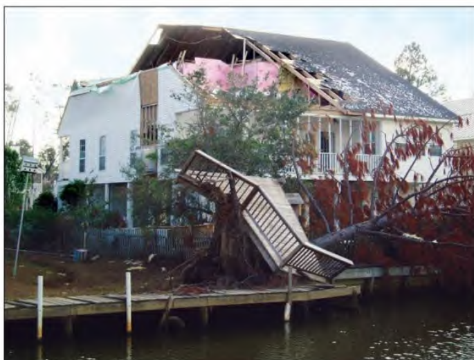
Figure 1-1. Wind damage to roof structure and gable end wall from Hurricane Katrina (2005) (Pass Christian, Mississippi).
