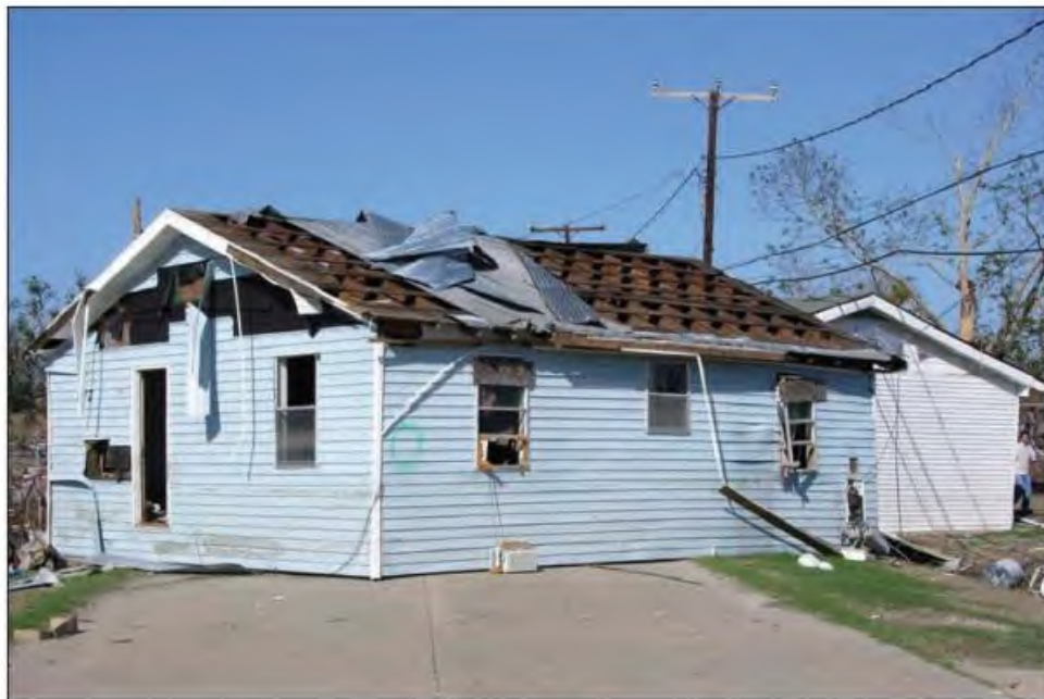
Figure 1-7. Building floated off of its foundation (Plaquemines Parish, Louisiana).
