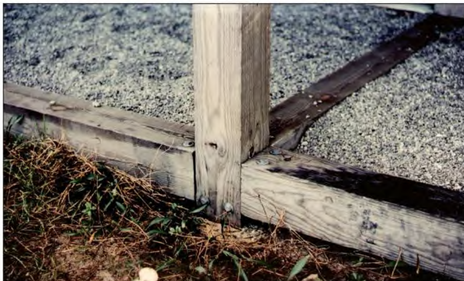
Figure 2-3. Compression strut at base of a wood pile. Struts provide some lateral support for the pile, but very little resistance to rotation.
